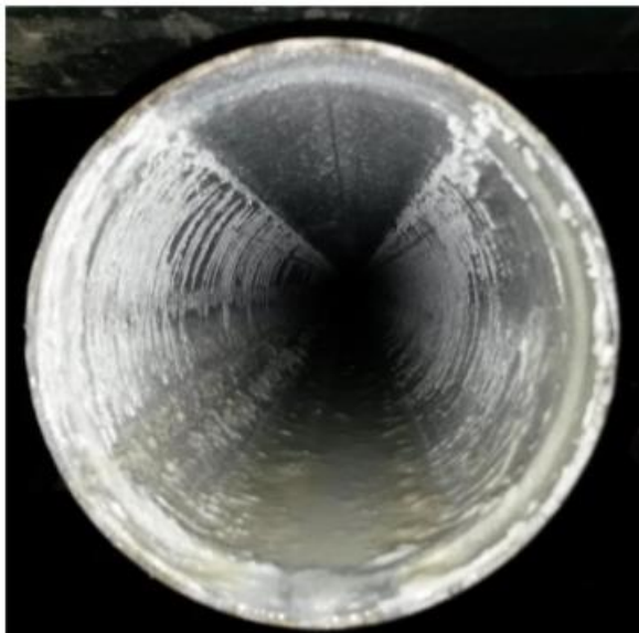
Picture 4 Galvanized pipe after draining on another system
