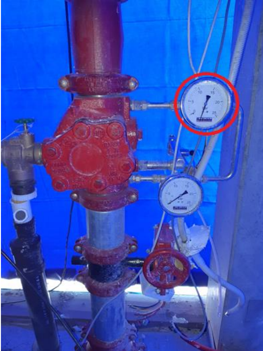
Picture 1 Control valve with manometer
