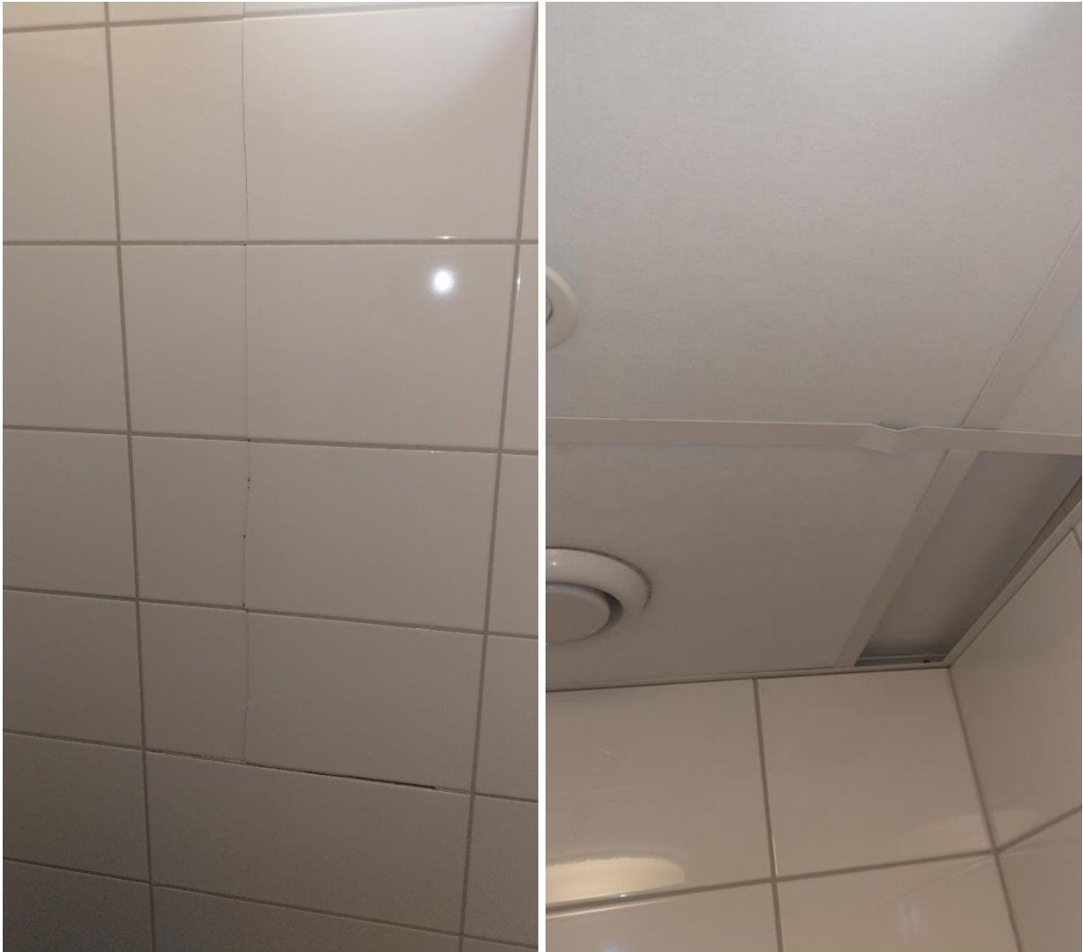
Picture 3 and 4 Damage tiles bathroom and ceiling
